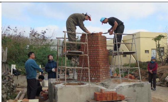
Excellent technical students of YunTech joined in the repair of fish stoves (chimney construction)
